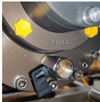
Closed Drain valve
