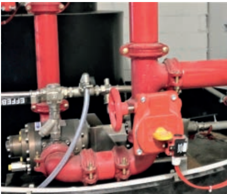
FM-approved FIREMIKS 1800-3-PP-F for Heli-deck protection at Hospital - Germany
